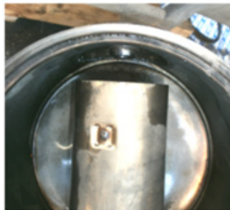
Use of Effinox prevents crystal formation and keeps the SCR system running.
